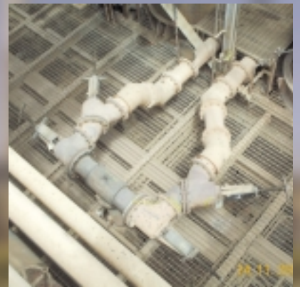
A typical piping system on the plant.
